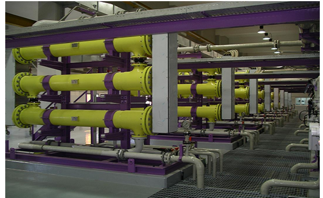
SEACLOR® Onshore Seawater
