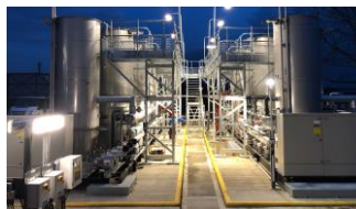
De Nora TETRA® mDBF Filters Southern Water, Tangmere WTW, UK
